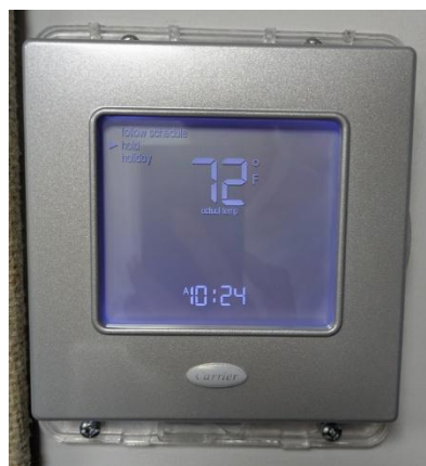
Figure 8: Thermostat for one of the old RTUs
