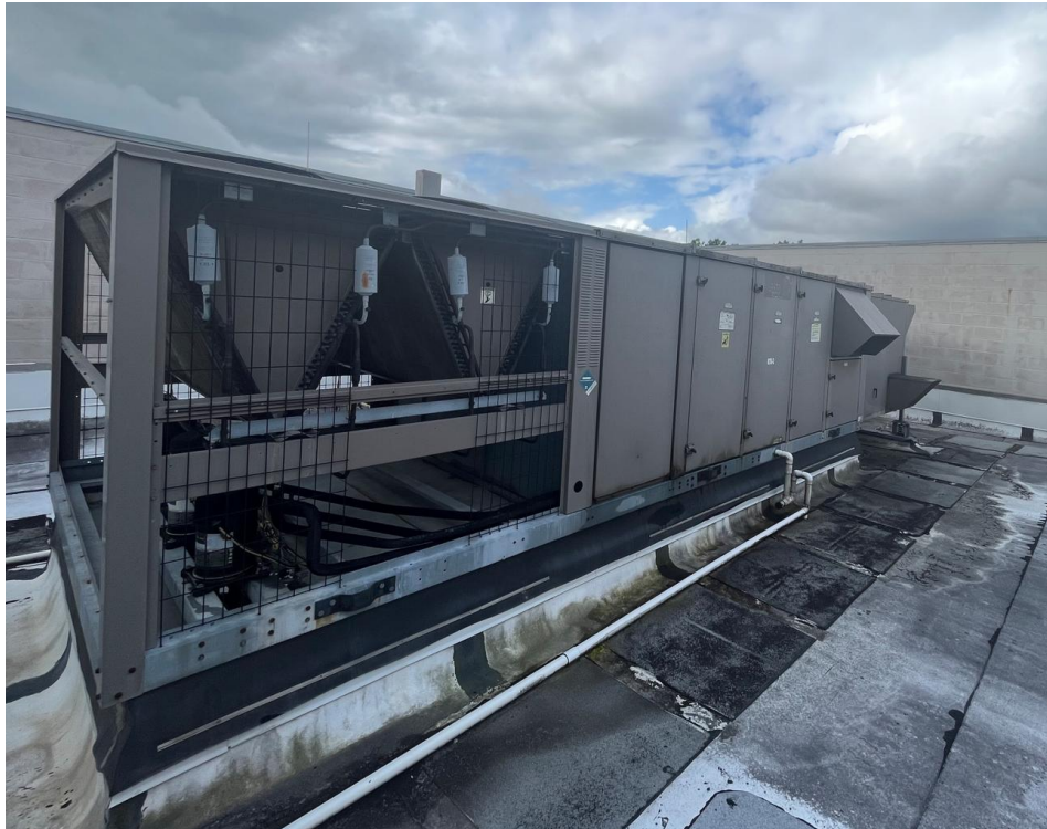
Figure 7: One of three rooftop units
