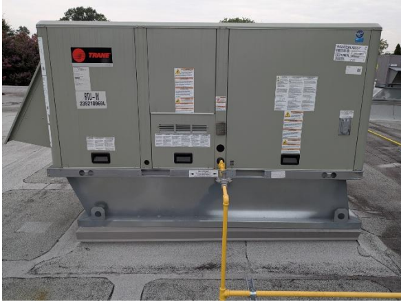
Figure 5: One of the new RTUs
