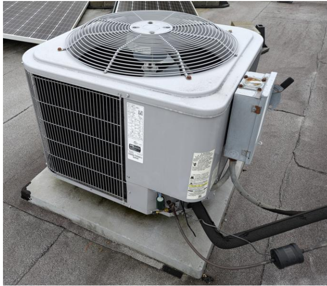
Figure 31: Condensing unit on roof
