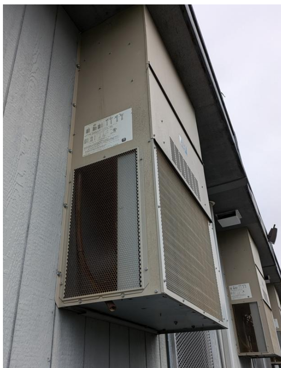
Figure 29: One of three wall-mounted air conditioners
