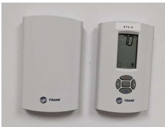
Figure 7: Thermostat for one of the new RTUs
