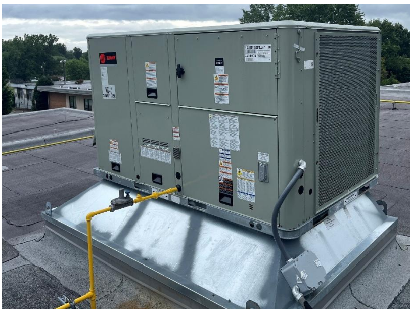
Figure 36: One of 28 gas rooftop units at Kenhill Center
