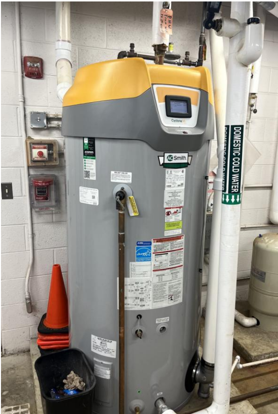
Figure 9: Domestic water heater
