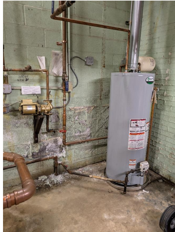
Figure 12: Domestic water heater and RCP
