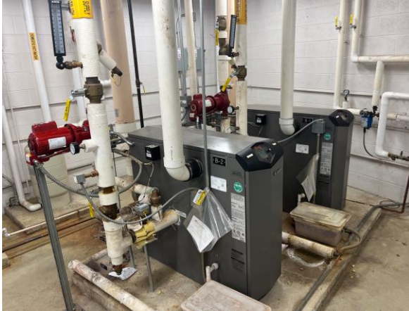
Figure 5: Hot water boilers
