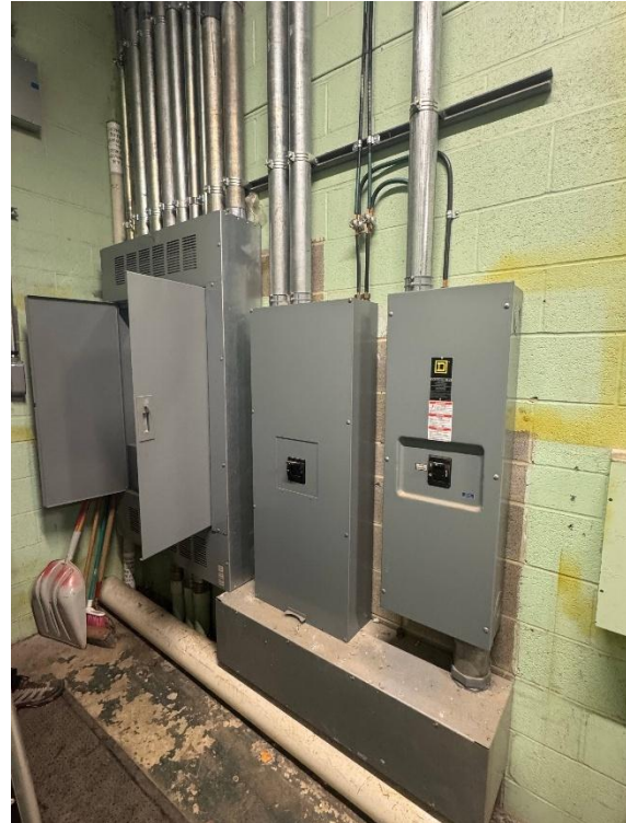
Figure 15: Main electrical service disconnects
