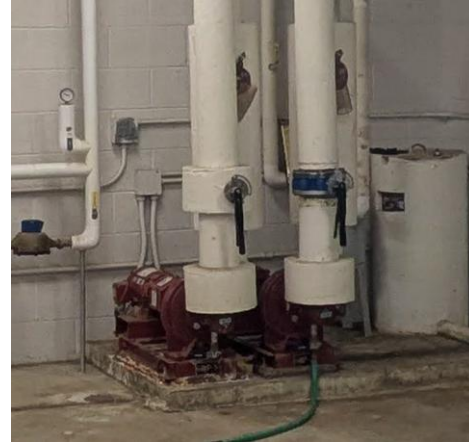
Figure 6: Secondary hot water pumps
