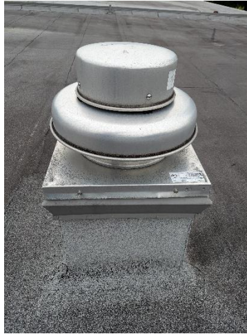
Figure 13: One of several roof-mounted exhaust fans
