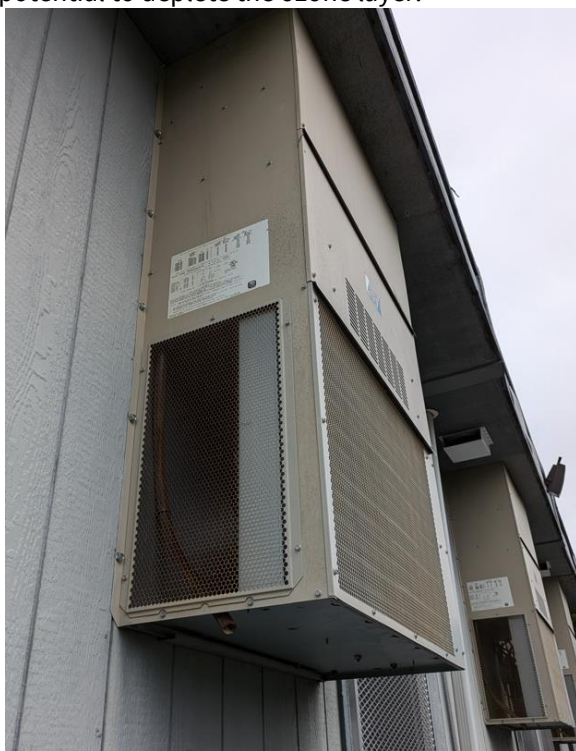
Figure 48: One of three wall-mounted air conditioners
