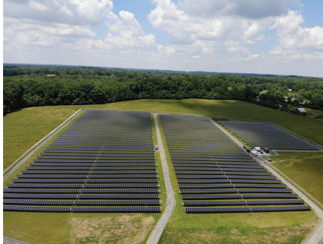
A photo of the City's solar farm.
